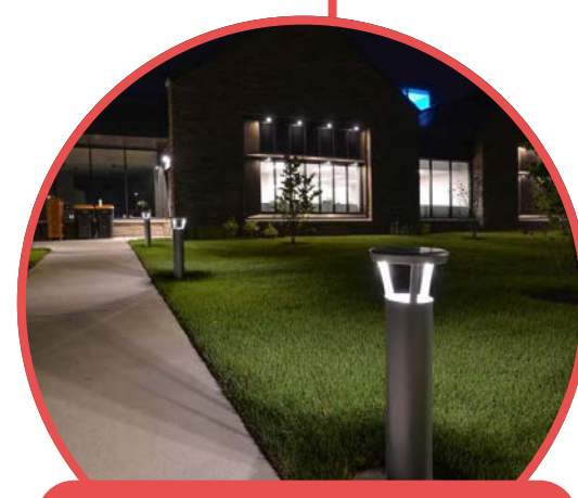
SOLAR BOLLARD LIGHTS
